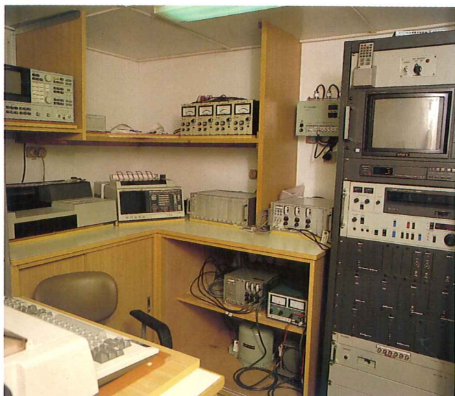
計測機器室 MEASURING EQUIPMENTS ROOM
